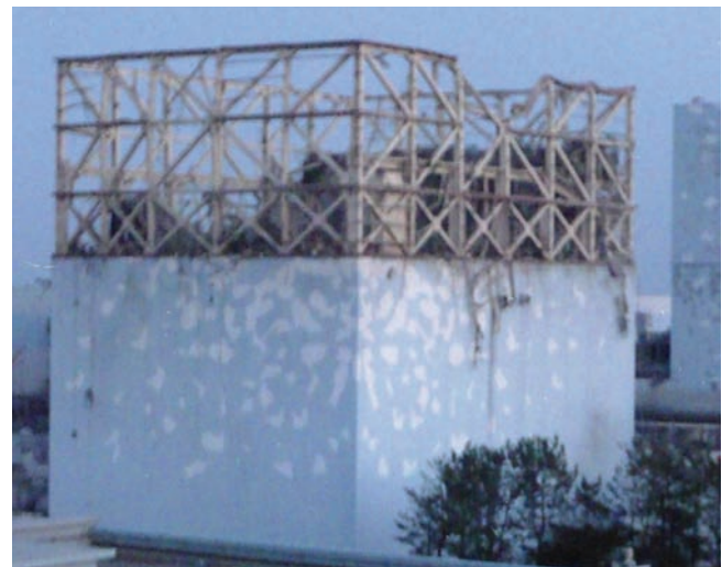
Unit 1 showing damage to secondary structures following hydrogen explosion on reactor service floor (© TEPCO)
